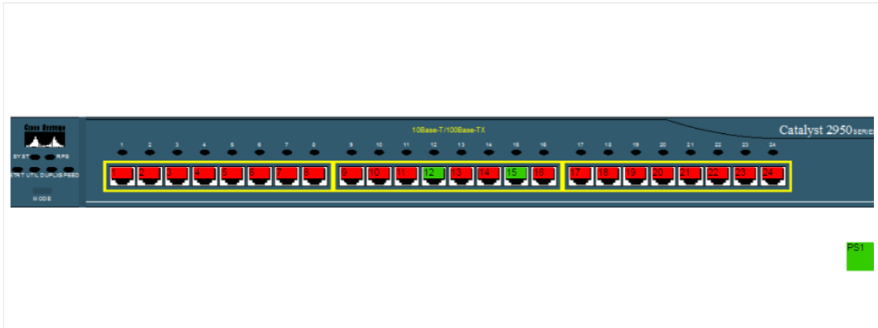
Port overrides based on operational status
